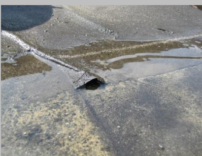
Slechte overlappen, loskomende dakbedekking
