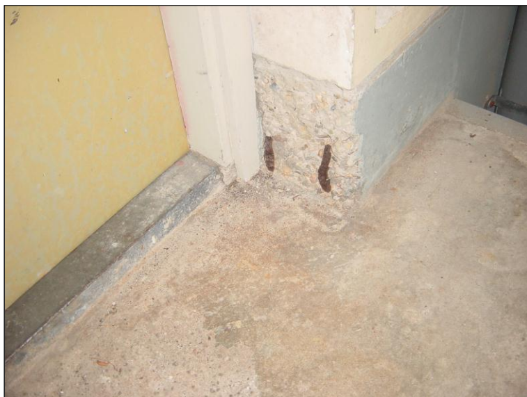
5. beginnende betonrot in betonplint
