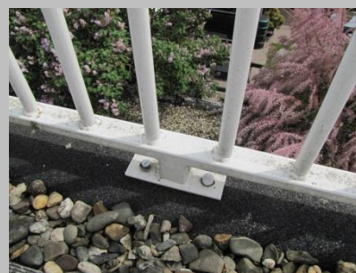
Loskomende verankering balustrade
